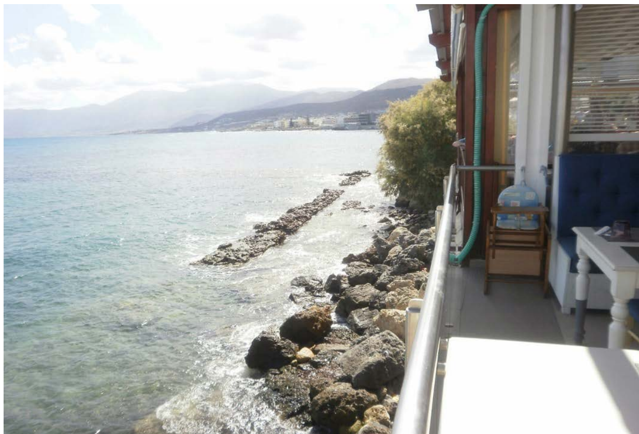
Figure 8.3. A section of partly submerged quay/sea wall at Chersonissos (photo by Michael J. Curtis).*
